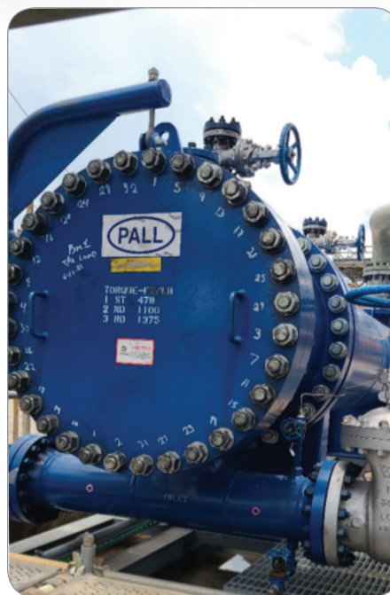
Photo showing one of two LL coalescer rental skids installed.
