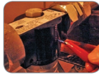
Discharge from filter housing to grounded alligator clip
