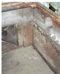
Corrosion in the reservoir
